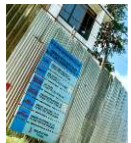
Plate 4.06: a construction of a multistorey hostel building in Sinza "A", Source: Author (2024).
