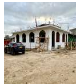
Plate 4.11: an on-going extension of multistorey Masjid Islamiya, without a signboard and stickers adherence to urban planning regulation, and without being registered by respective regulatory bodies, i.e., AQRB, ERB, CRB, OSHA and NEMC, Source: Author (2024).
