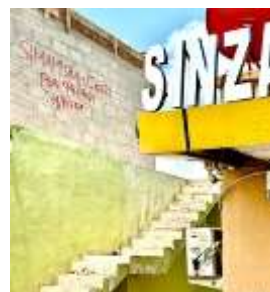
Plate 4.10: an on-going building project without LGA's building permit, unregistered by respective regulatory bodies (i.e., AQRB, ERB, CRB, OSHA and NEMC) and a signboard and stickers, leading to an estoppel for an extension of a multistorey commercial building in Sinza "A", Source: Author (2024).
